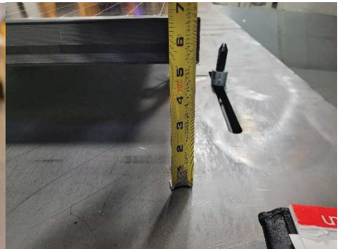
Figure 6: Height from roof to panel, Runs 2 & 3
