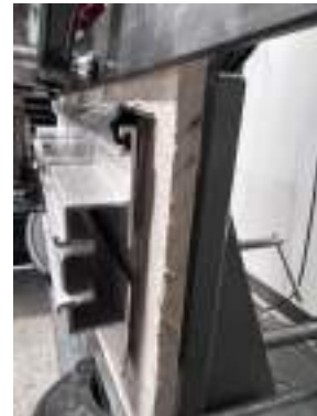
Photo 12: De-bond between the aluminum to adhesive interface
